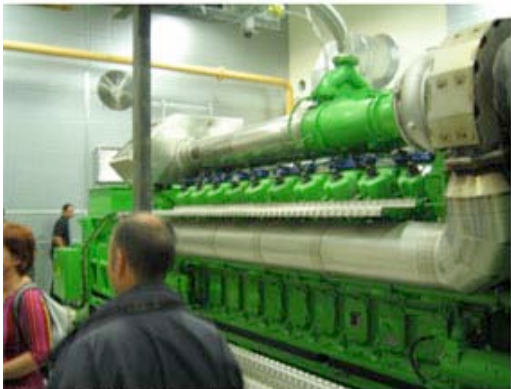
The CHP Engine
